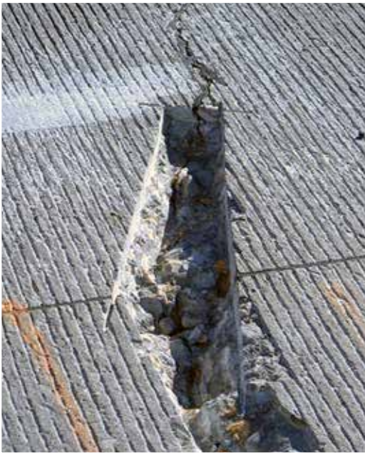
Pot hole in concrete highway
